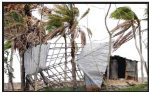
The wind is blowing the roof away.
